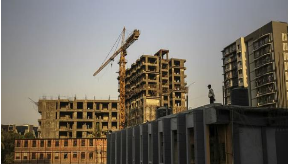
Abandonment of ongoing construction sites
